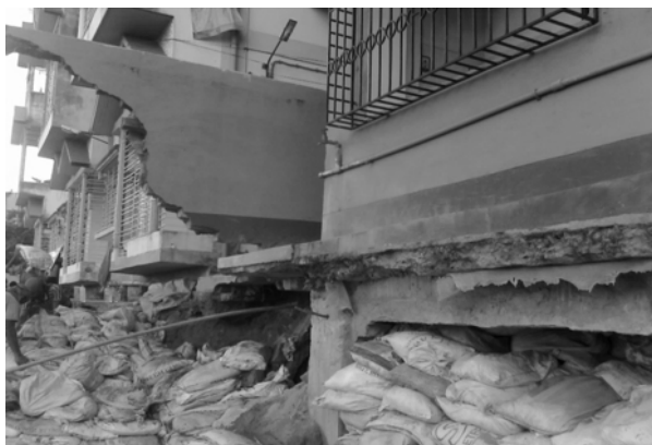
Ganges Valley Apartment badly affected
