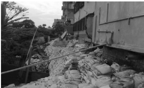
Affected Red Cross Building
