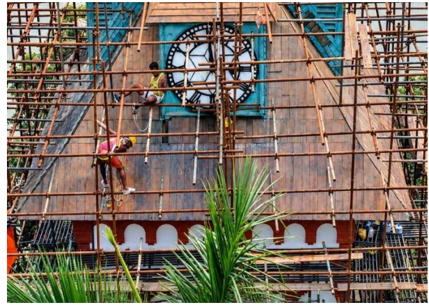
Photo-2 Condition of 1 st layer timber after removal of the upper layer timbers
